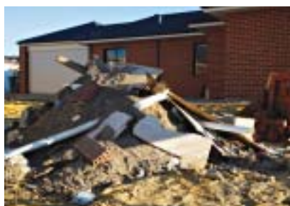
Typical building site with poorly managed waste. (Source: EarthCare Recycling)
