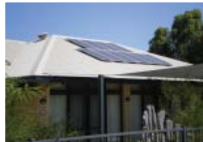
Solar PV system generating power from the sun (Source: Sustainable Mandurah Home)
